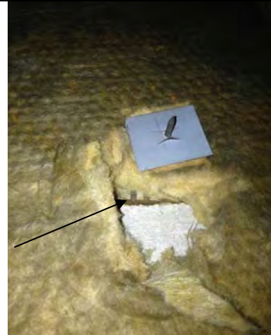
4. 1714 2 nd St: View of Brown Pin Mastic (ACM) associated with Fiberglass Insulation in the 2 nd Floor Conference Room. Sample No. BS-28.
