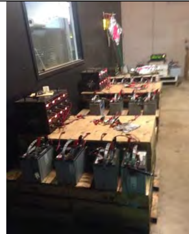
14. 1714 2 nd St: View of Batteries in Garage.
