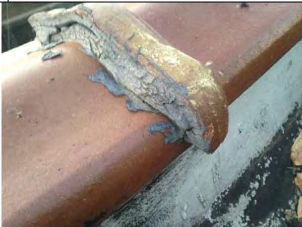
21. 1711 1 st St: View of Gray Copping Stone Caulk (ACM) on the Roof. Sample No. SSR-13.
