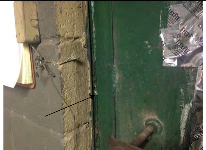
16. 1711 1 st St: View of Gray Interior Window Caulk (ACM) in the Rear Office. Sample No. SS-05.
