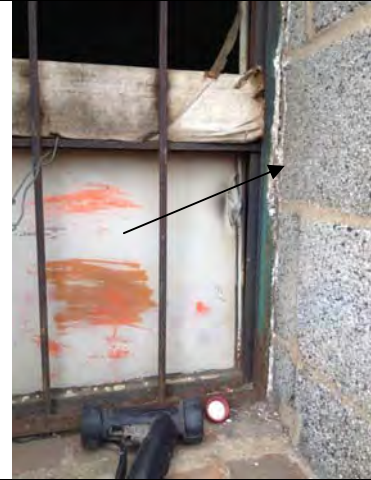
20. 1711 1 st St: View of White Exterior Window Caulk (ACM). Sample No. SS-19.
