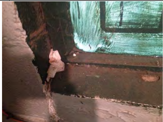
17. 1711 1 st St: View of White Interior Window Glaze (ACM) in the Rear Office Bathroom. Sample No. SS-07.
