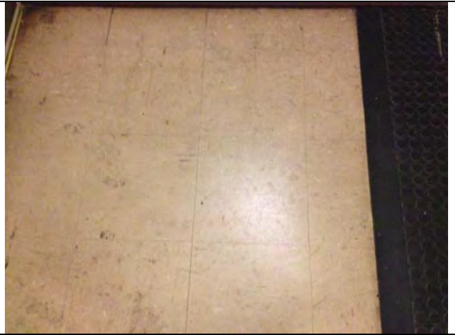
2. 1714 2 nd St: View of 12" x 12" Tan Floor Tile (ACM) in the Stairwell. Sample No. BS-9-A.
