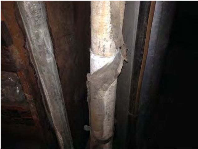
19. 1711 1 st St: View of Pipe Insulation (ACM) in the 2 nd Floor Storage Area. Sample No. SS-15.
