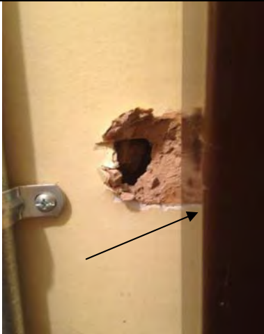
3. 1714 2 nd St: View of Drywall Joint Compound (ACM) associated with Brown Drywall in the 2 nd Floor Closet. Sample No. BS-13.
