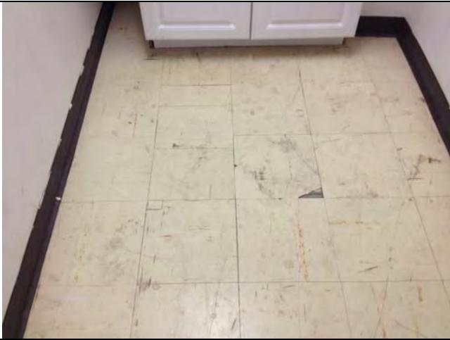
1. 1714 2 nd St: View of 12" x 12" Off-White Floor Tile (ACM) in the 2 nd Floor Kitchen. Sample No. BS-5-A.
